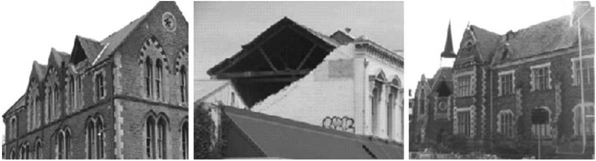
Figure 3. Typical damage to gable walls in the September 2010 earthquake.
