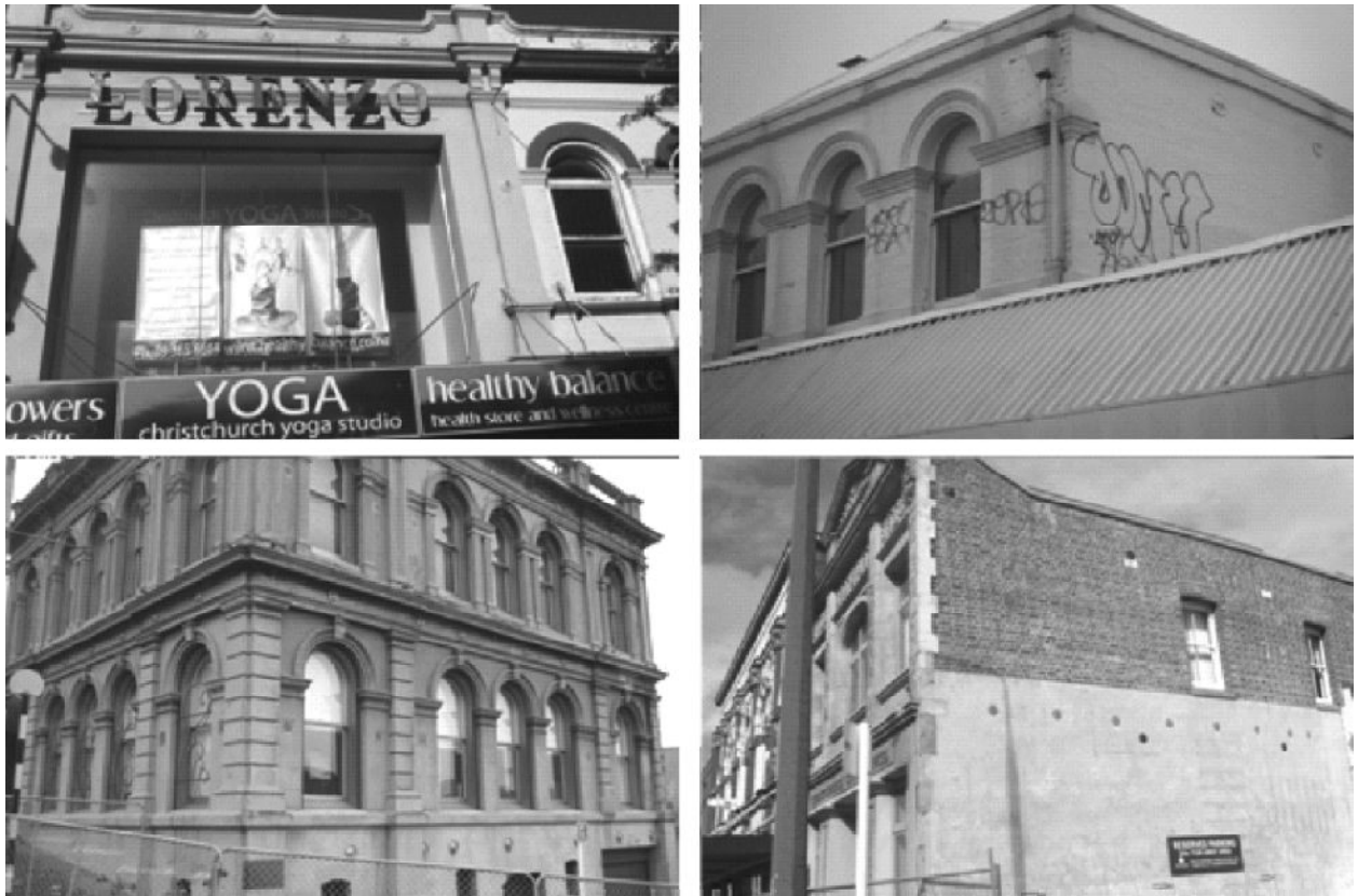
Figure 22. Good performance of some URM buildings with anchored perimeter walls in the February 2011 earthquake.
