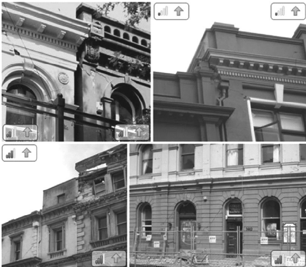
Figure 20. Building pounding damage observed in the February 2011 earthquake (Photos: Greg Cole).
