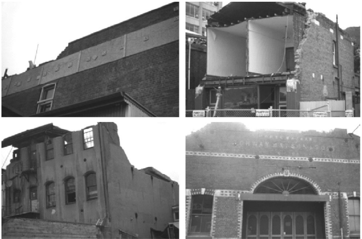
Figure 23. Damage to systematically anchored masonry walls in the February 2011 earthquake.
