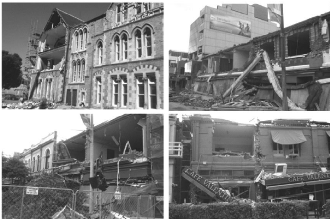
Figure 16. Failure of gable walls and parapets observed in the February 2011 earthquake.
