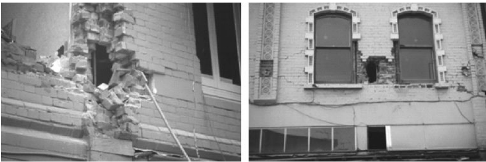
Figure 18. Punching failure of masonry walls due to inadequate anchorage (February 2011 earthquake).
