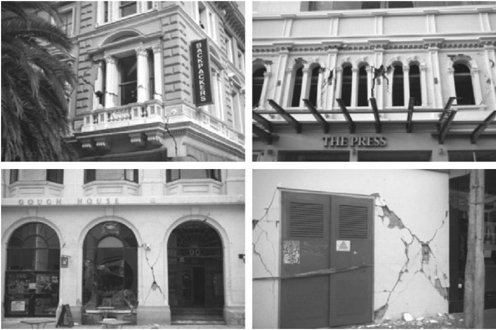
Figure 17. In-plane damage to walls/piers/columns/arches observed in the February 2011 earthquake.
