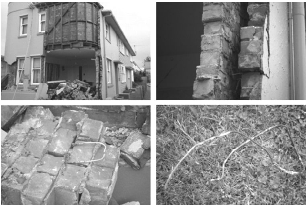
Figure 19. Failure of cavity walls due to inadequate ties (February 2011 earthquake).
