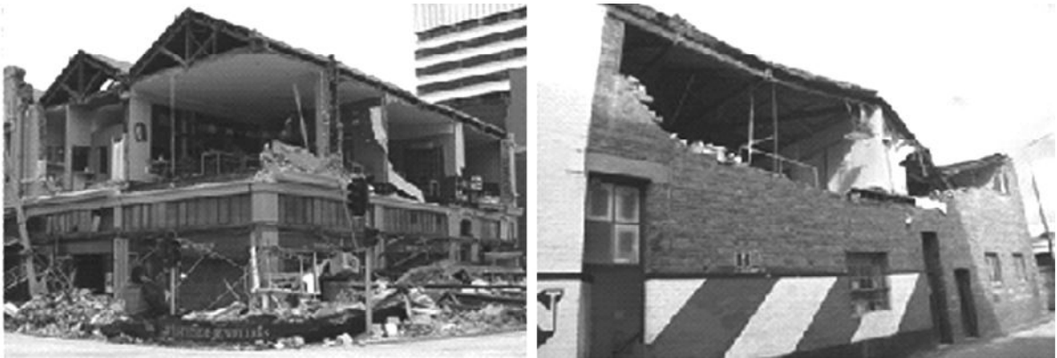
Figure 4. Typical out of plane failure of solid masonry walls in the September 2010 earthquake.
