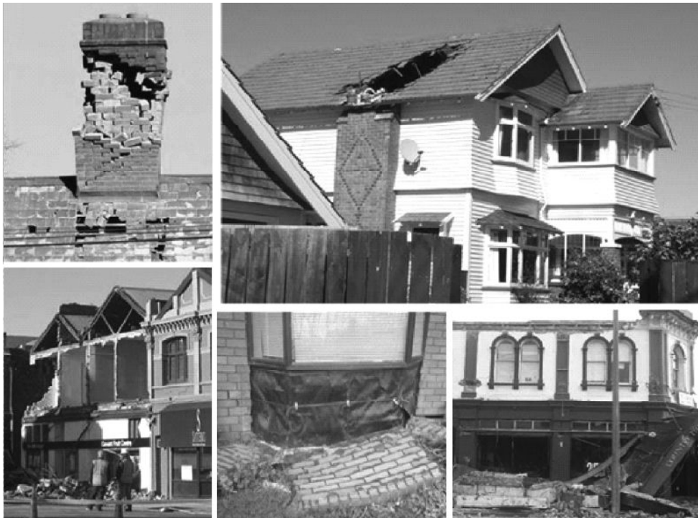
Figure 8. Failure of brick masonry chimneys, facades, walls and parapets observed in the September 2010 earthquake.
